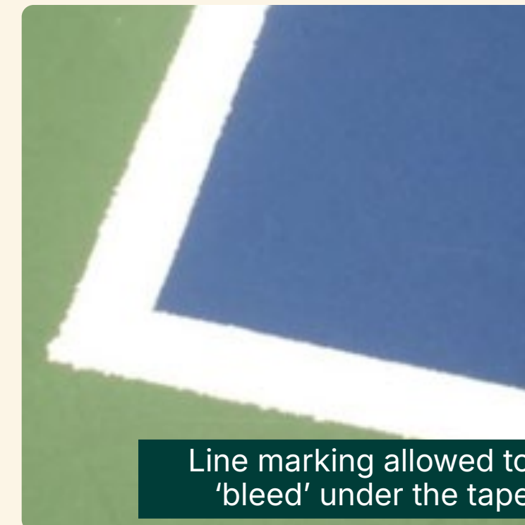
Asphalt damage due to use of oil-based paint
