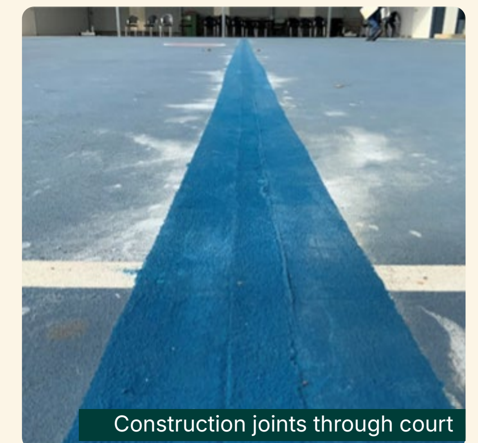
Concrete joints – tripping hazards
