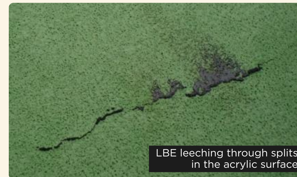
Cracked court filled with liquid bitumen emulsion
